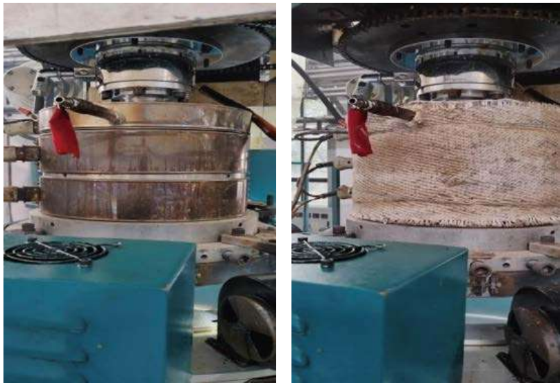
Exposed heating equipment (left) and heating equipment with insulation layer (right)
